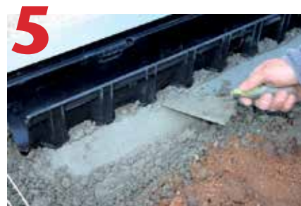
5 Lay 4" deep concrete bed. Lay channels working away from outlet. Concrete surround should extend up channel sides into recesses to hold channel in place.
