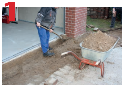
Excavate area to allow room for channels/catch basin and 4" of concrete on all 3 sides.
