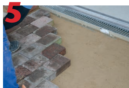
Install pavers or finish pavement surround to required level. Should be 1/8" above grate.
